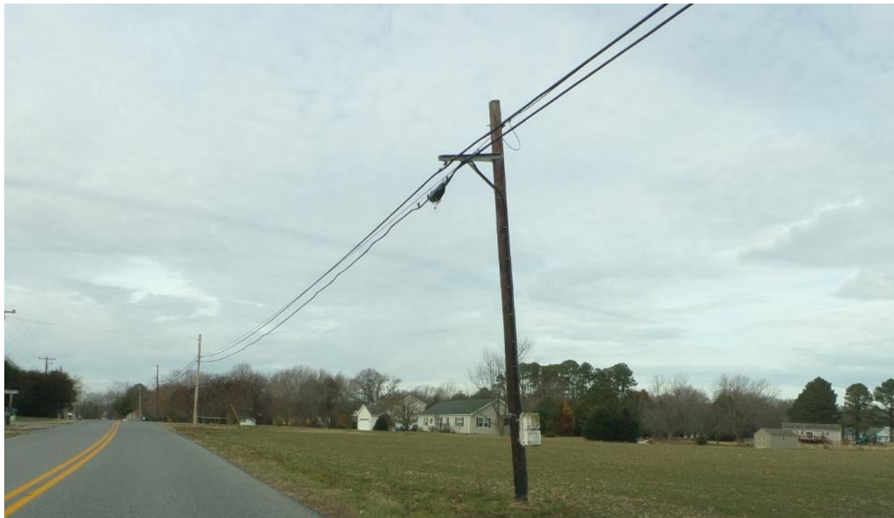
Figure 16: Utility Pole Requiring Make-Ready
