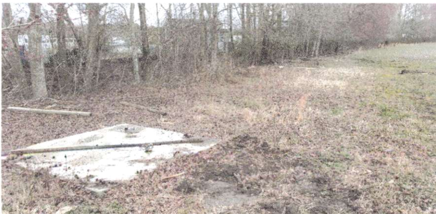
A silt fence will be installed along treeline/ditch to prevent any sediment from entering ditch.
