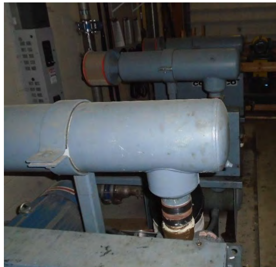
Photo 4: Membrane Blowers – Add Dip Tank Blower
