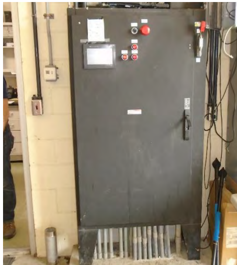
Photo 5: MBR Control Panel – to be Replaced
